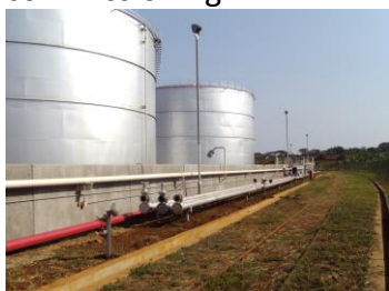
Figure 58: The facility in Jinja has started operation
