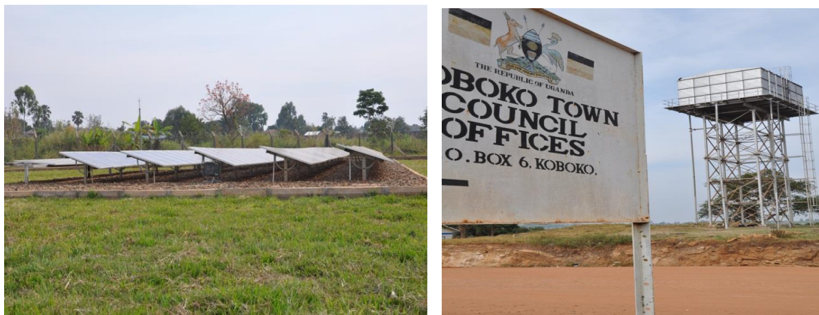
Figure 16: (left): Solar Array at Koboko Water Station; (right) The scheme's 100,000m 3 capacity reservoir tank
