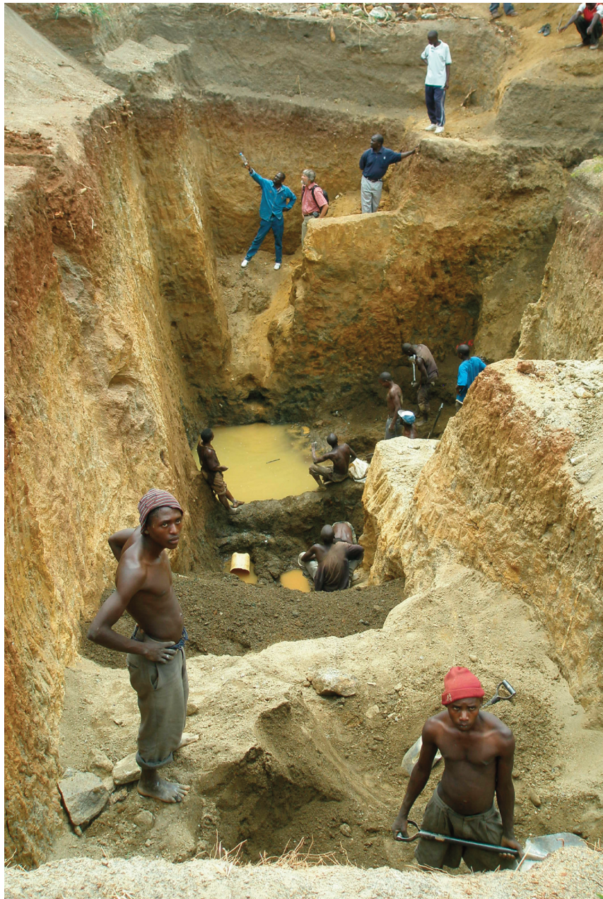
Fig. 7-10. Very deep pit with near vertical walls with a high risk of accidents caused by falling stones.
