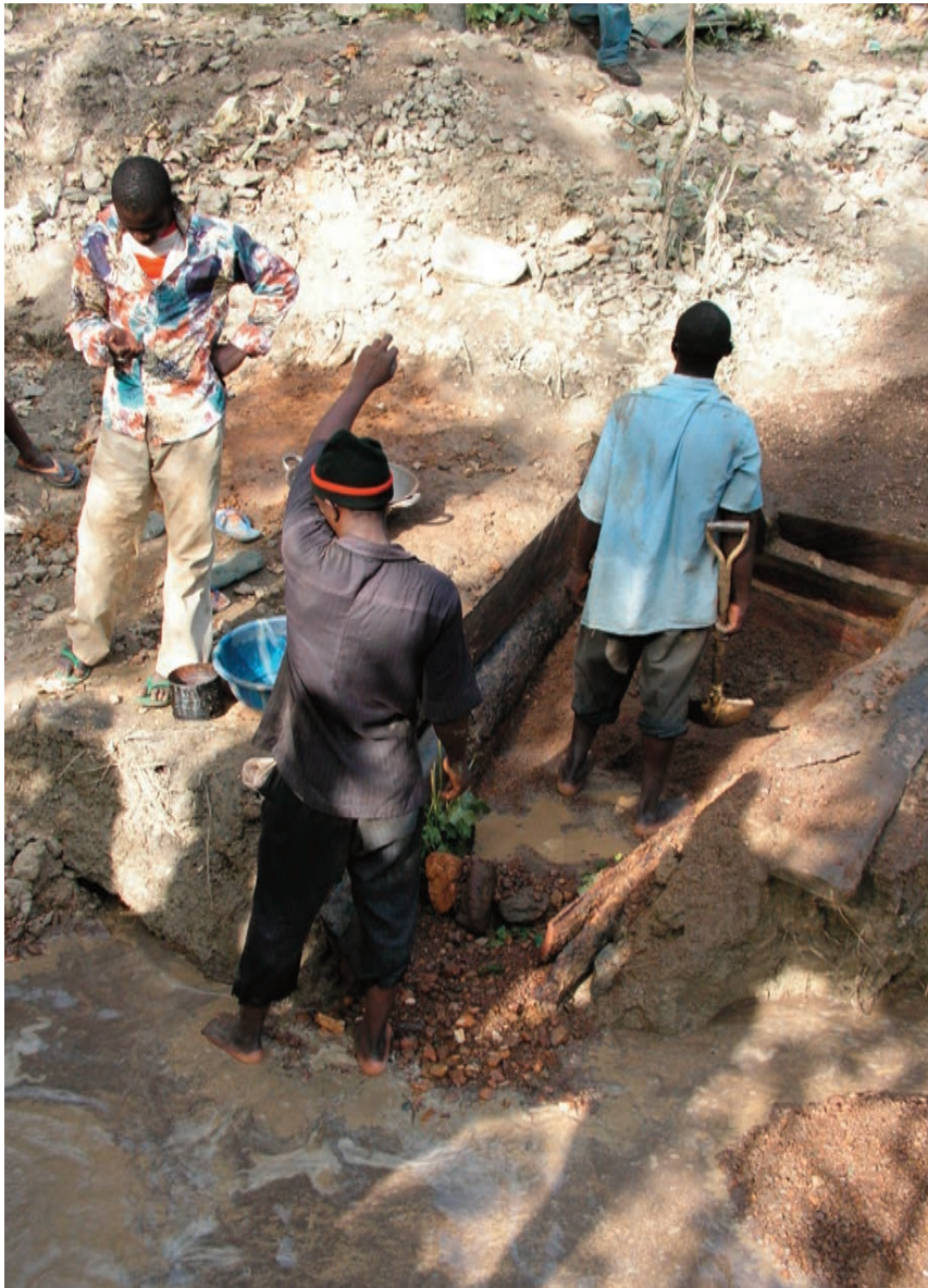
Fig. 6-1-A. A very primitive sluice where buckets of water are thrown on the upper part of the sluice. The result is that many of the heavy mineral grains (gold or tantalite) will be washed out of the sluice and get lost at Tongakura, Kogi State.
